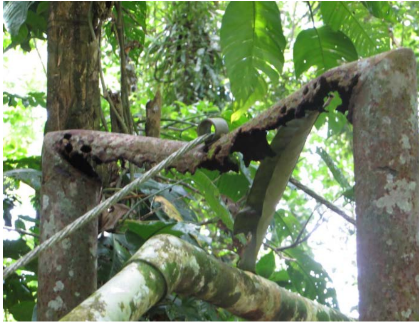
Figure 12: Degraded Metal Support
